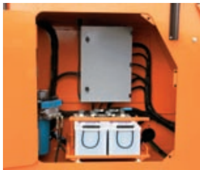
Service hatch on right hand side. The batteries can be rolled out.
